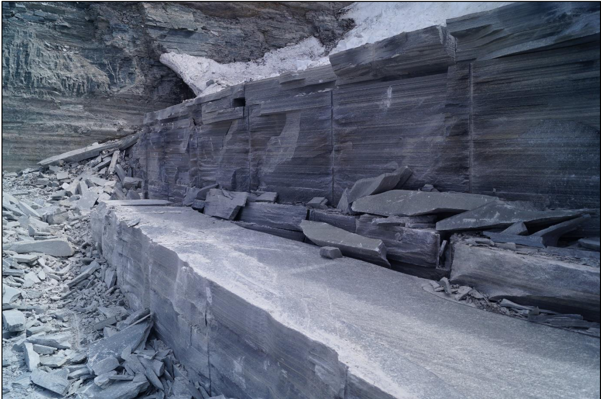
Figure 8. After blasting. Explosives employed in spaced, vertical drill holes defining a surface line along the rift of the schist. No need for horizontal drill holes, since the rock will loosen along the “plane of weakness), i.e. schistosity/cleavage plane. On the far side of the photo, a fracture along the grain defines a natural border for blasting.
