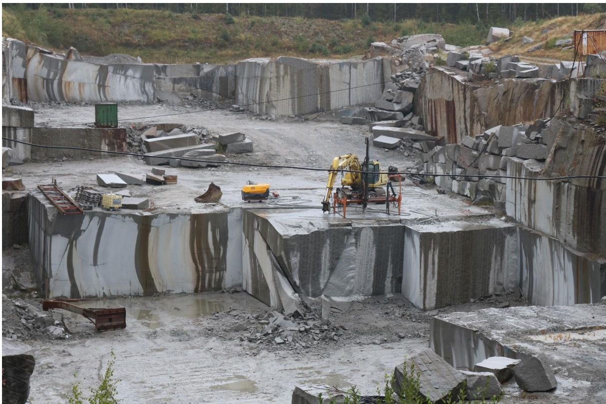
Figure 14. Diamond wire sawing of two surfaces (horizontal and vertical perpendicular to photo plane) and drilling/blasting of one direction (vertical parallel to photo plane)
