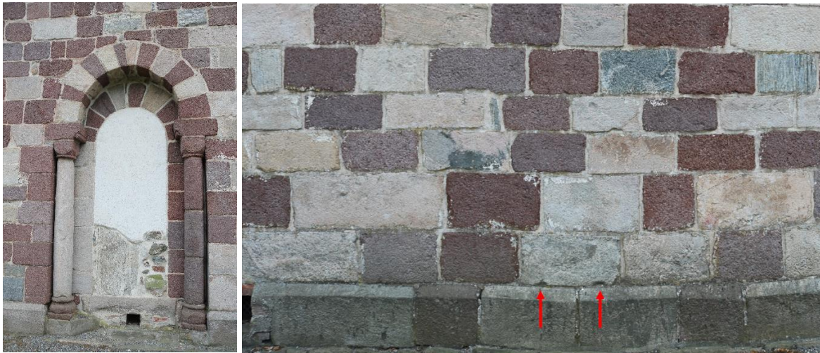
Figure 10. Rygge medieval church polychrome portal (left). Stones in the portal: Iddefjord granite (grey), oxidised monzonite from the western Oslofjord area (brown) and local, Precambrian gneiss (banded). Right: Wedge holes in granite ashlar (red arrows)
